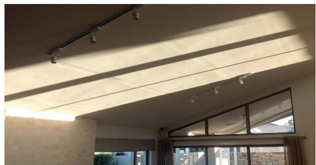
Figure 8: Same Plasterboard Surface Under Glancing Light
