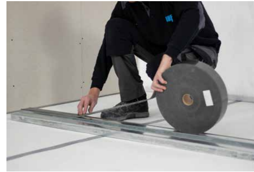
Provide all profiles connecting to the surrounding building elements with Knauf Sealing Tape.
