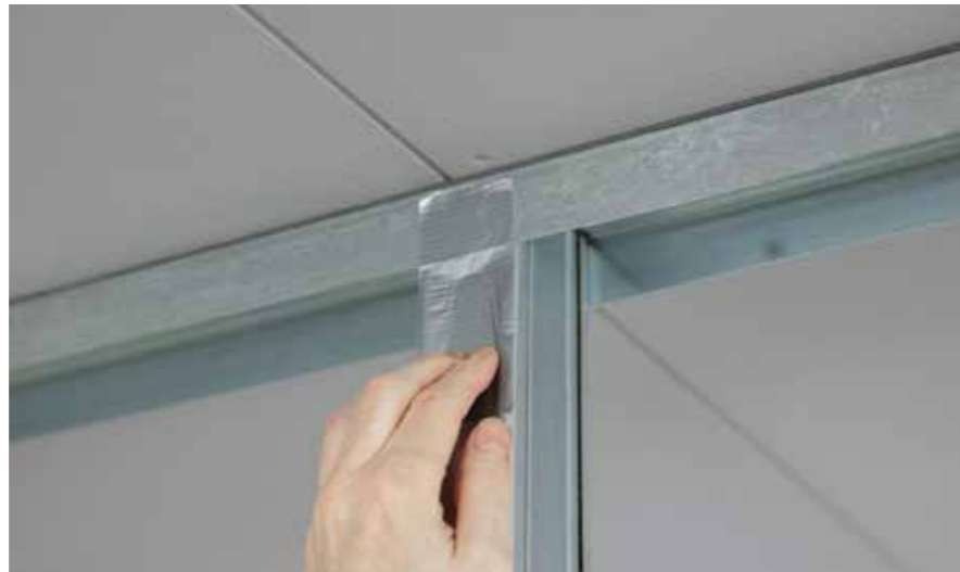
Temporarily fix the Knauf MaxSpace uprights to the UW profile with duct tape.
