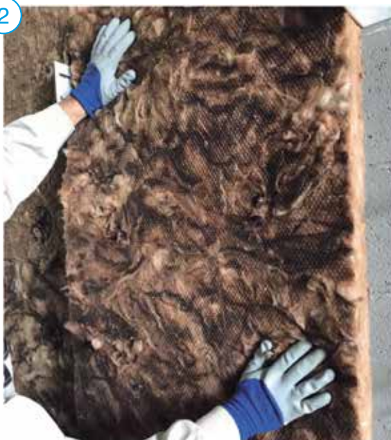
Placing and fixing the thermal insulation to the wall of support. Mineral wool must be placed accordingly.
