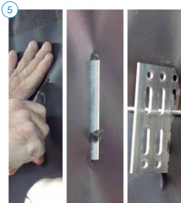
The waterproof membrane is placed. It is cut by the height of the bracket and temporarily fixed with a locking element. Later it will be held.
