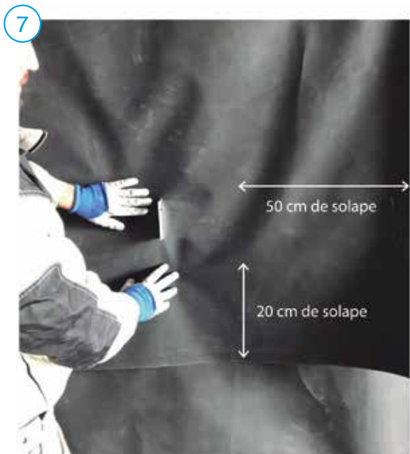
Overlap the membranes 50 cm vertically and 20 cm horizontally according to water flow direction.
