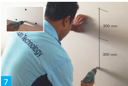
7 Install the gypsum board using a 25 mm gypsum screw fixing to the installed metal profile on every 300 mm along the C Stud (avoid the screw on the metal profile on the both end) then every 200 mm around the edges.
