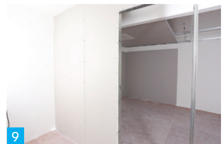
9 After the gypsum board installation, check the screw head. If it is exceed the gypsum board level, use a screwdriver to make it even.
