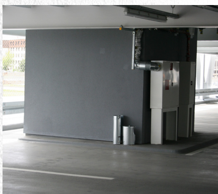
Car Park Utility Rooms | Stuttgart, Allemagne
